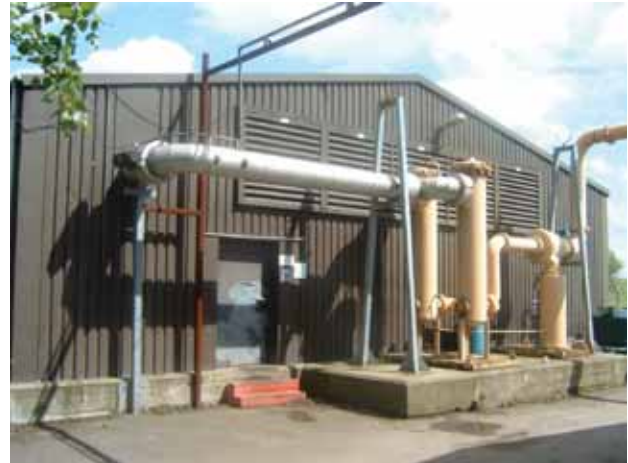
Aveley Methane Plant
